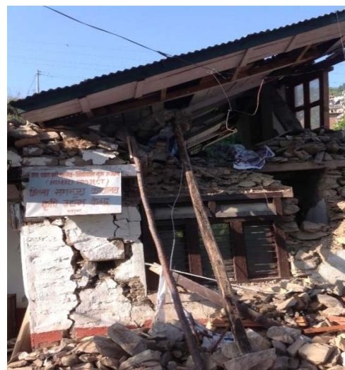
Figure 4: Damaged rural agriculture service centre
